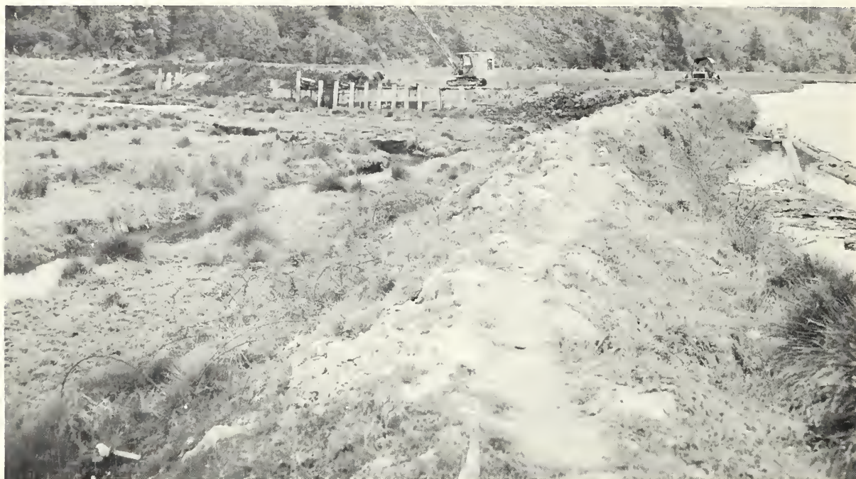
Photo 27.--An inadequate dike and tide gate is being repaired after damage from high water, North Fork Siuslaw River, Oregon, 1963. SCS photo NO. 7-1391-12
